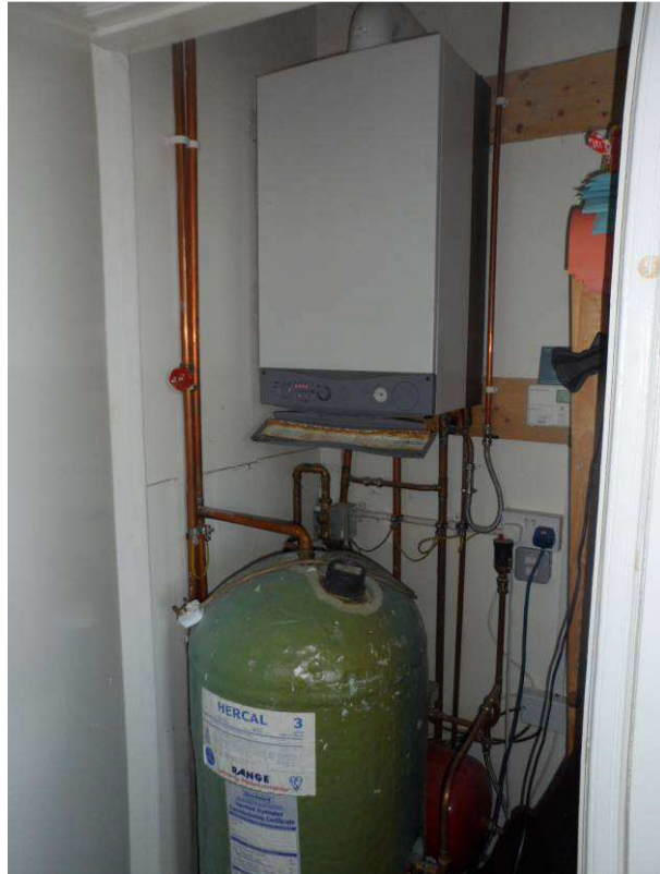
View of boiler and hot water cylinder
