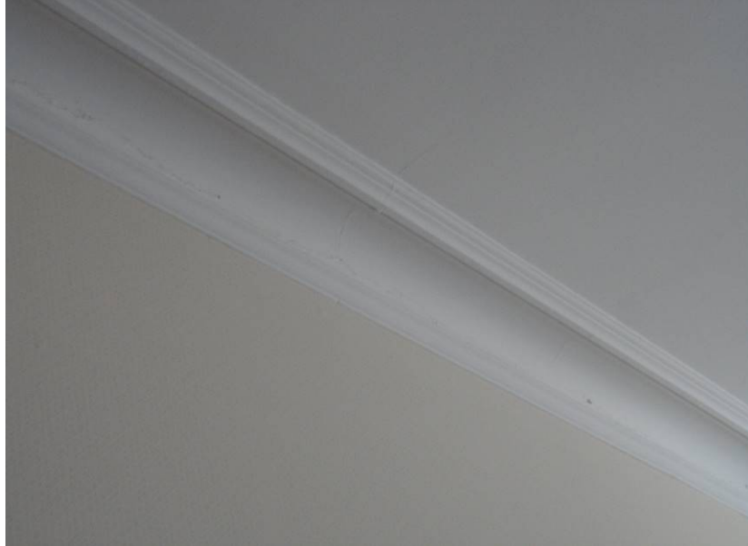
View of cracking to cornice in the lounge
