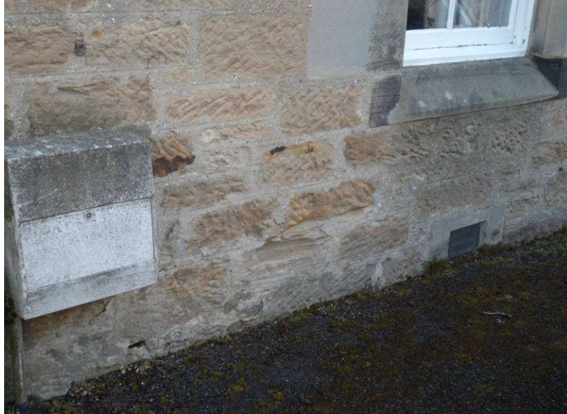
View of typical erosion to stonework
