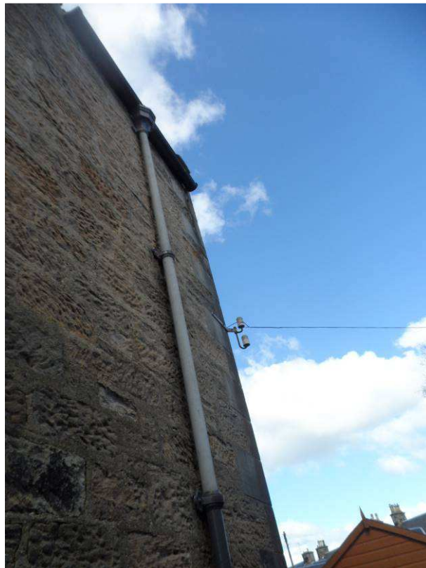
View of unpainted downpipes
