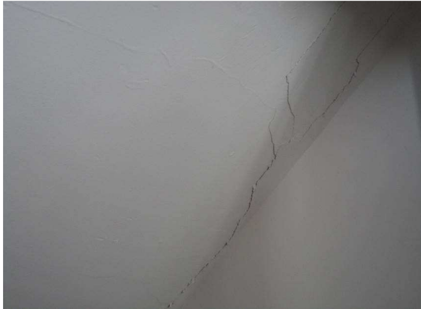
View of cracking under stairs in entrance cupboard
