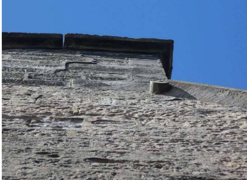
View of movement to east chimney stack
