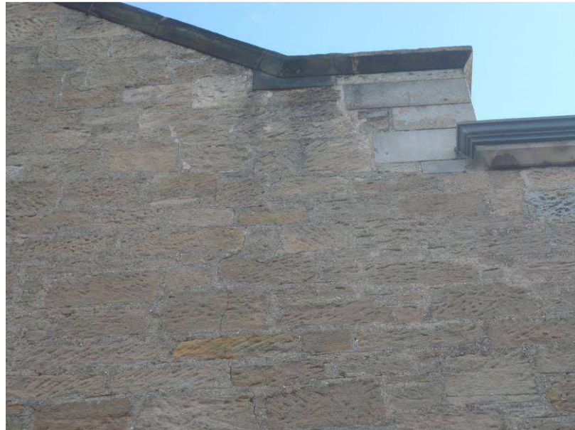
View of minor cracking to west elevation
