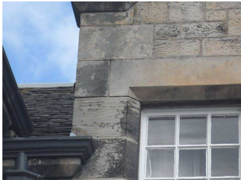
View of missing pointing to front elevation
