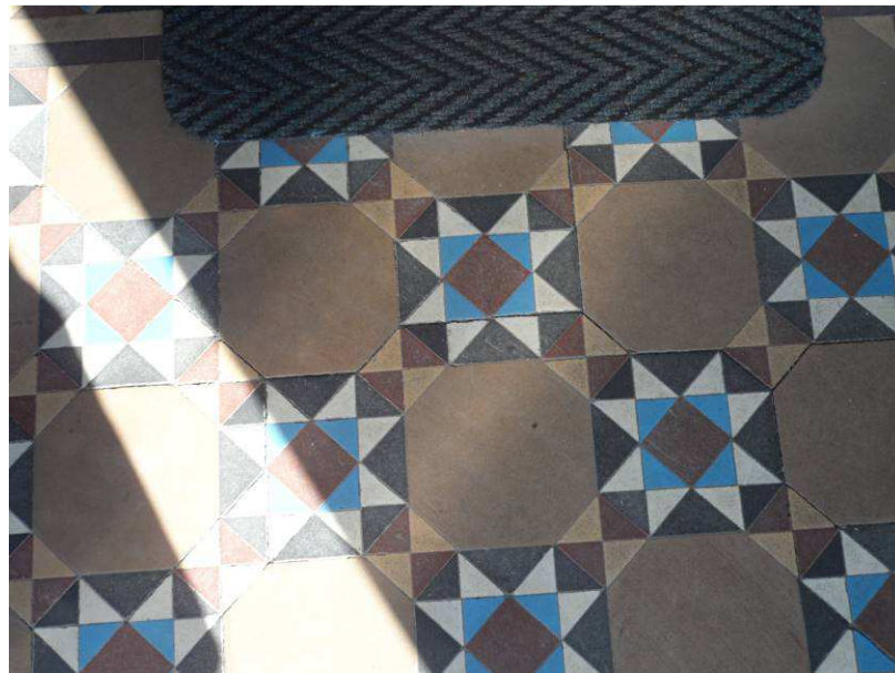
View of missing grout to tiles at entrance door
