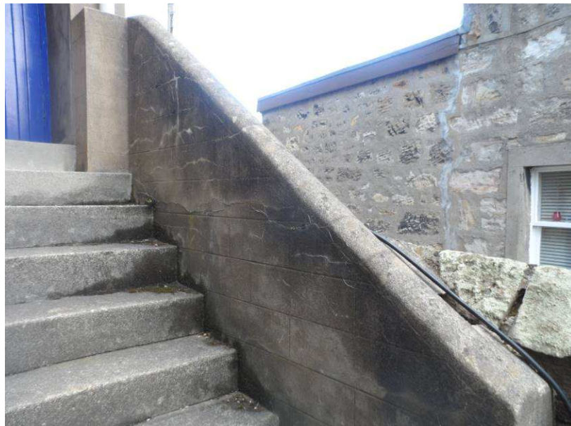
View of cracking to smooth render at steps to front elevation
