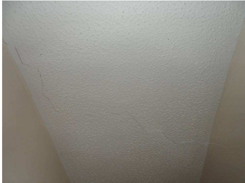
View of cracking to ceiling within entrance hall
