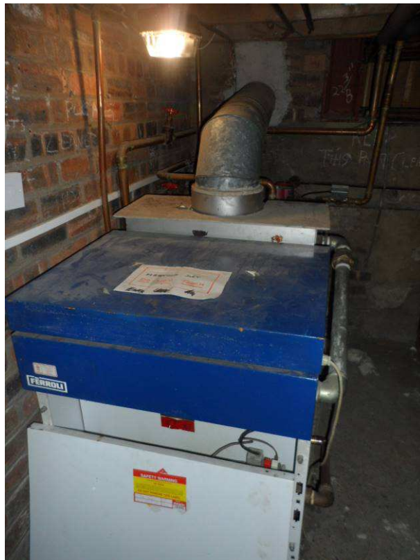
View of current boiler system
