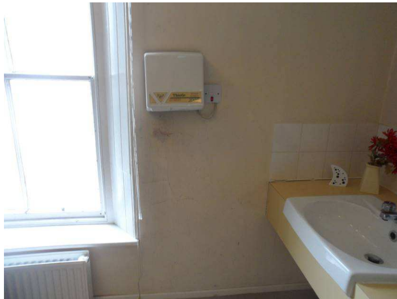
View of deterioration to wall decoration from hand drier used in Ladies WC
