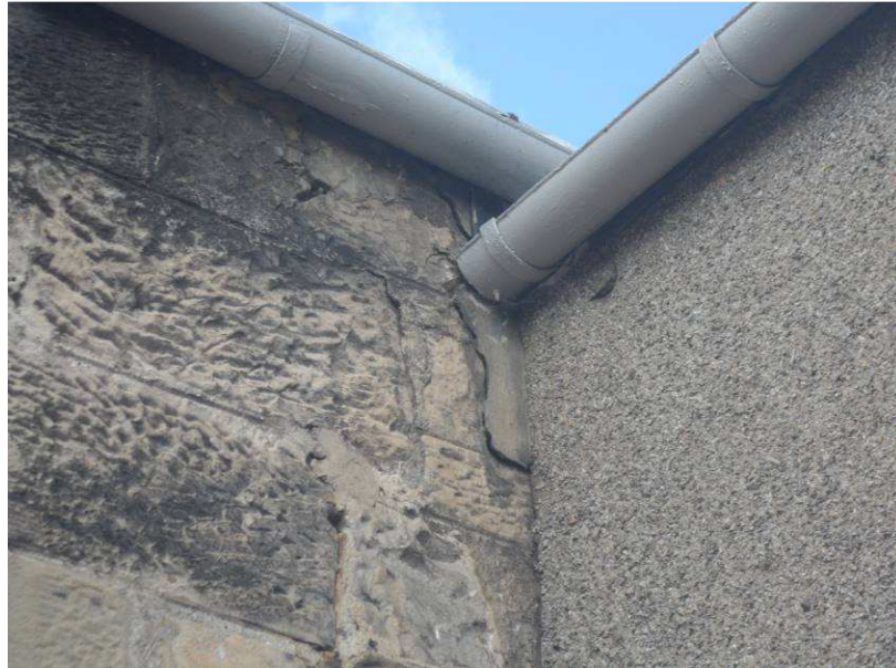
View of cracking to front elevation
