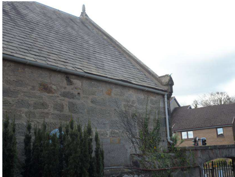
View of uplift to slates
