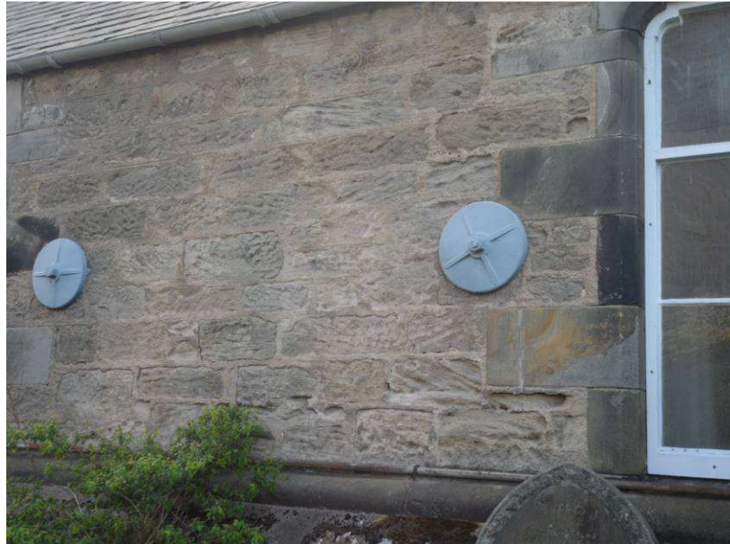
View of typical stone erosion
